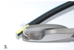
3. Pull out the conductor and cut it of. Be sure that non of the core stick out or can get in touch with the other conductor
